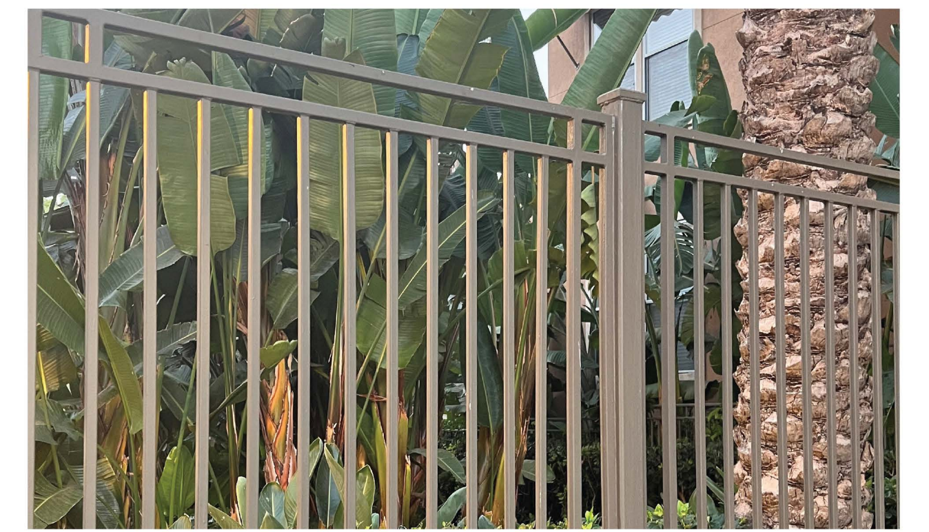
TUBULAR STEEL FENCING
